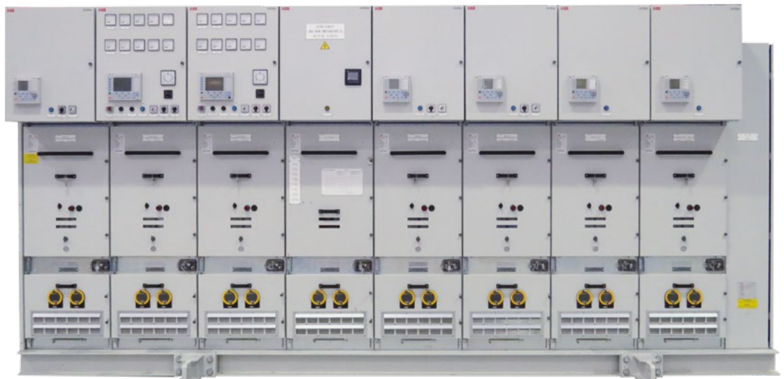
Main Switchgear with withdrawable circuit-breaker panels type LSC2B
